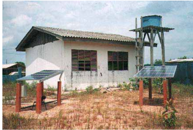
Pumping system and health center
