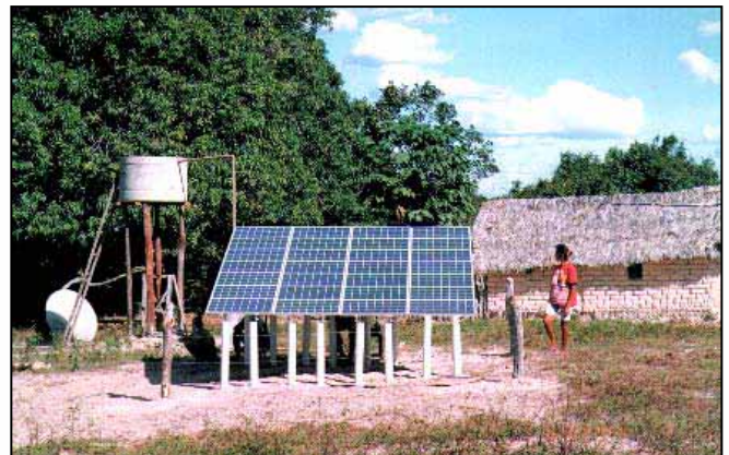
Small farm pumping system
